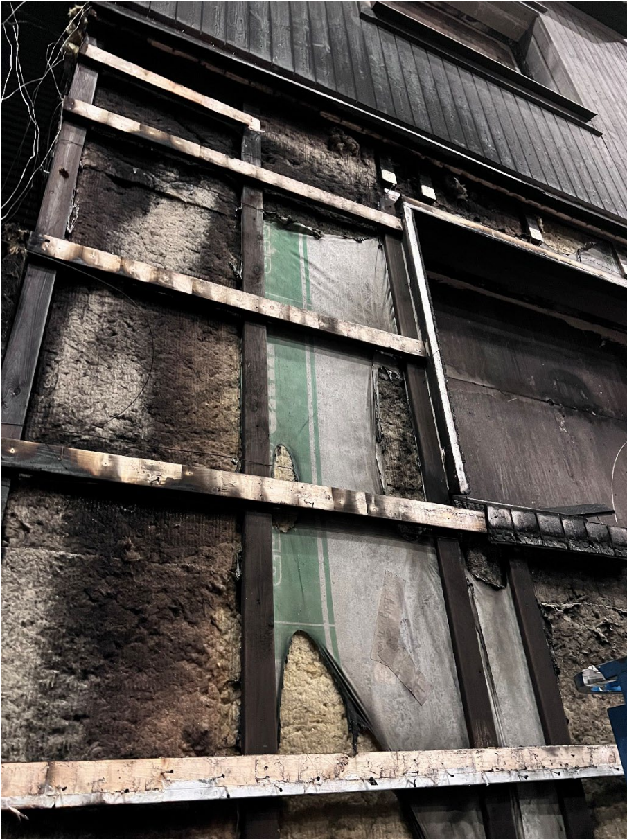
Photo A- 5 Close up of the lower part of the test specimen with the cladding removed.
