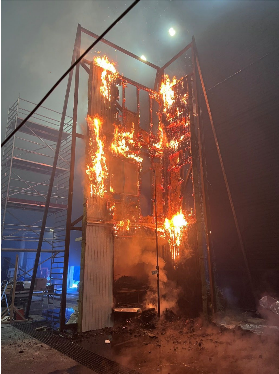
Photo B-8 Overview of the test specimen after the crib has been extinguished.
