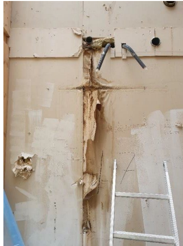
Figure 15 - Moisture damage around pipes that were cut in connection with disassembly.
