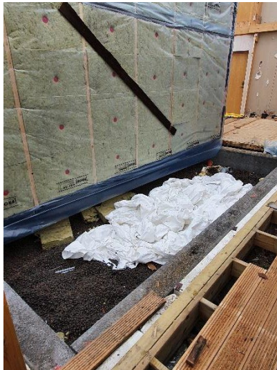
Figure 23 - The parts that did not have a basement floor were built on a crawl space.
