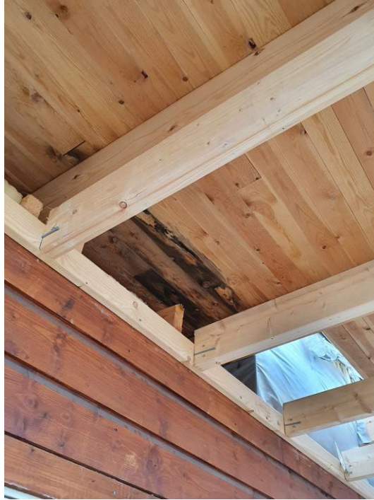
Figure 7 - Moisture damage to the roof of the staircase/ access balcony.
