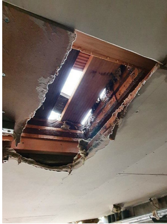
Figure 9 - Moisture damage in staircase ceiling.
