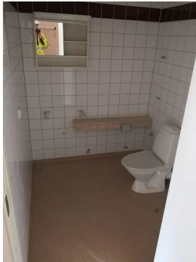
Figure 12 - Bathroom in apartment. Sinks, pipes, and mixer taps were stolen from all apartments in connection with a burglary.
