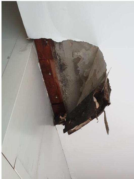
Figure 8 - Moisture damage in staircase ceiling.
