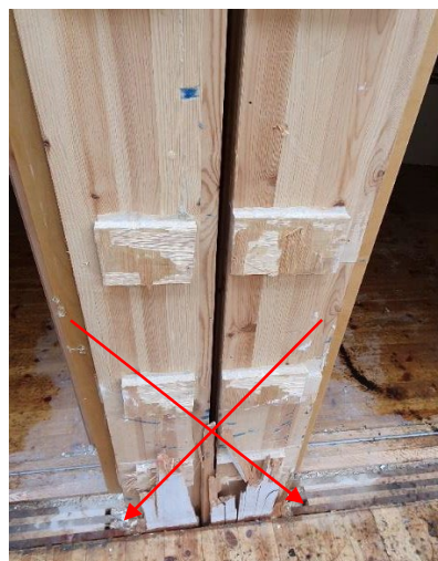
Figure 13 - Joint between two apartment modules. The arrows illustrate how the modules were screwed together, which made deconstruction more difficult.
