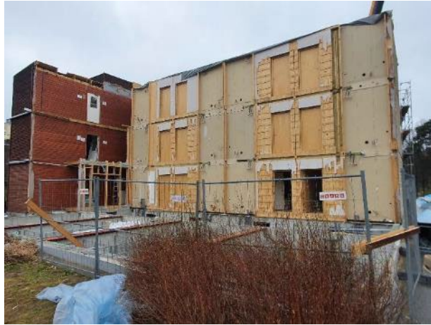
Figure 22 - At the time of our investigation, there was no plan for the basement structures after dismantling.
